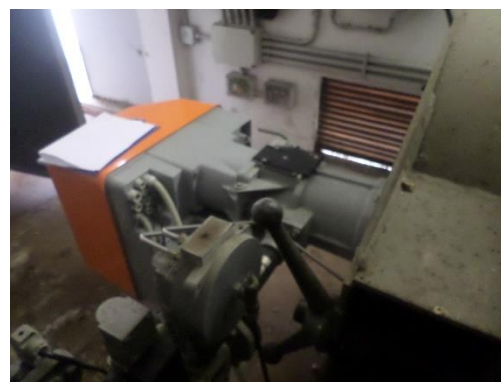
Figura 4.16 - Boiler a gas
